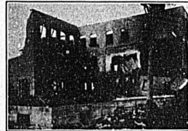
Two views of the wreckage of the Ghiglione macaroni plant. Nothing but the walls remain of the 4-story reinforced concrete and brick building, while the tall chimney alone remains to mark the spot occupied by the power house. Plans are being prepared for rebuilding, the work to start immediately.
